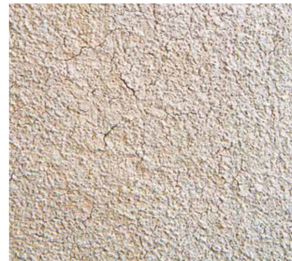
(1) A dry and clean cracked surface
