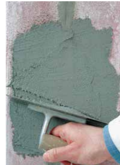
(4) Total leveling treatment with a coat of rialto intonal or mixture based on rialto matonal
